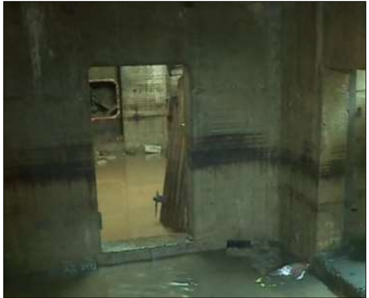
Pictured: The flooded bunker in Middlesbrough.
